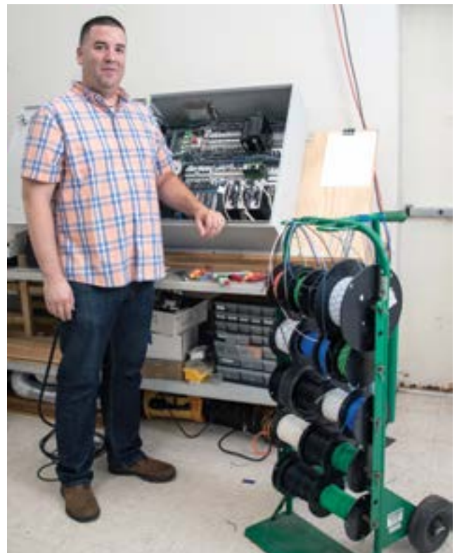
Adam Carlock just completed assembling and wiring the connections for the build station used to make the electronics box and panel. The box holds the electronics for the build and is pressurized to keep the explosive vapors away from any components that could spark. The unit is built to control 3 "slave units".
